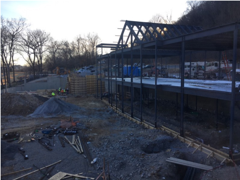
The new fitness center and pool area under construction at Richland Country Club on Dec. 12.
